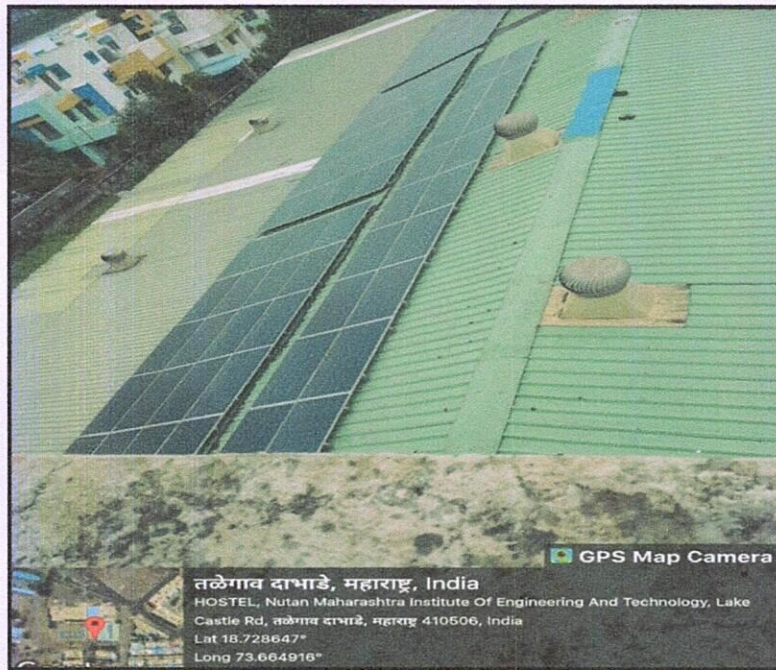
Photograph of Roof Top Solar PV Plant:
