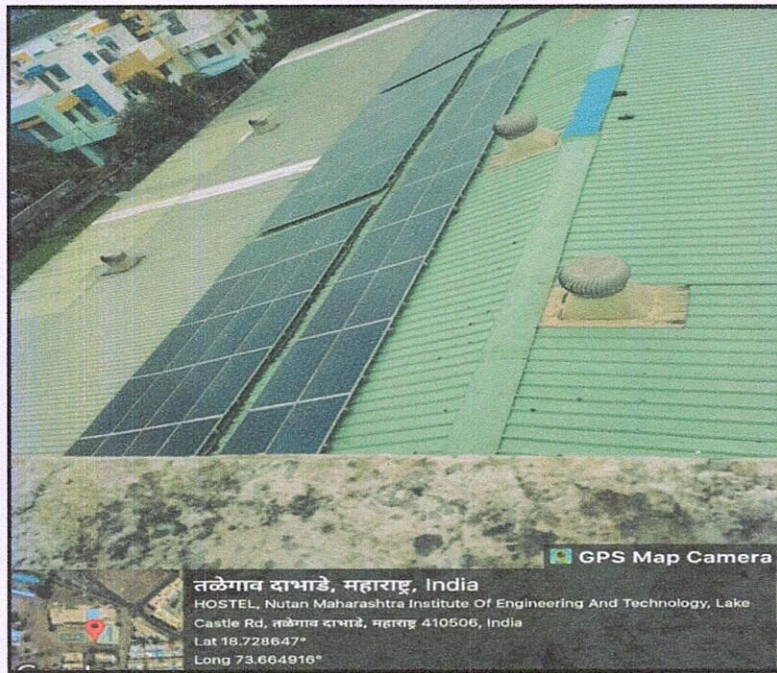
Photograph of Roof Top Solar PV Plant:
