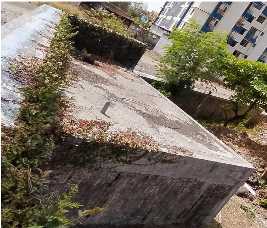
Rain water Storage Tank
