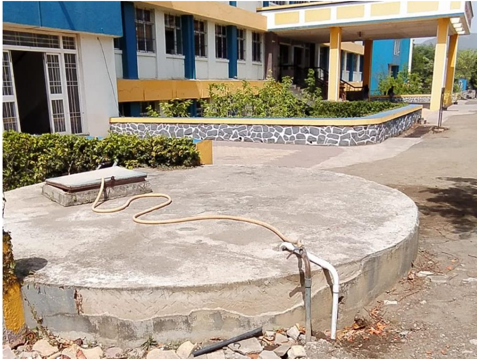
Well maintained storage tanks
