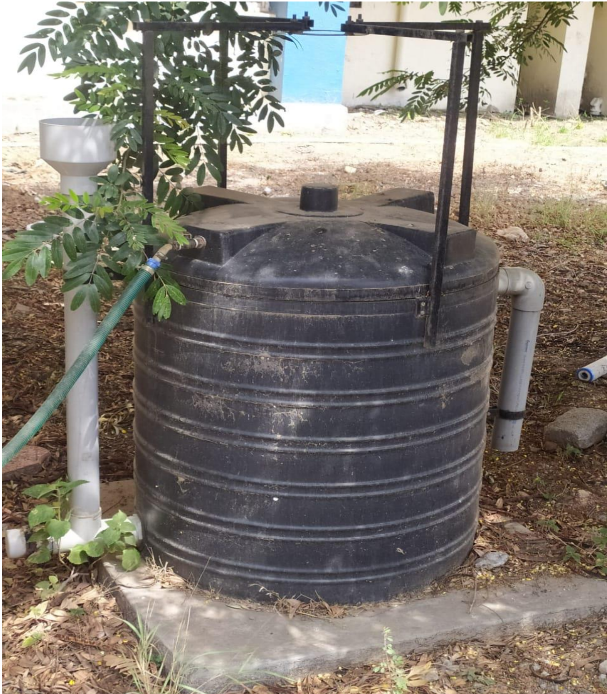
Canteen Waste Biogas Plant
